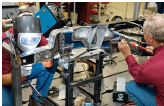
Tom Sefried joins in the fun as the team nears the completion of the front frame modifications. At this point, final welding has taken place, and all the component pieces are being welded together. Just study this shot for a moment and appreciate all the hand work and fabrication—and we're just looking at the front of the frame.
