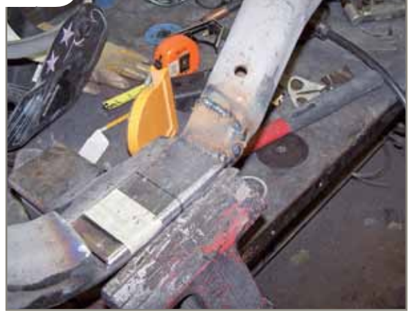
Welding side pieces in place provides a strong support for the transmission. Although an aftermarket crossmember might be available, it was quicker to modify the one we had.
